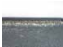
Thermal Cracks (Thermal Wear)
